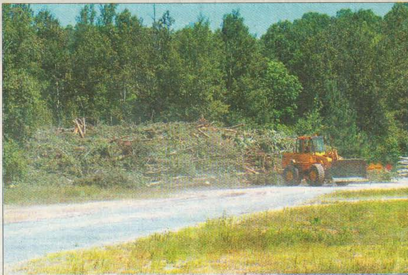
The remains of many fine trees are piled in the Radcliffe Number 2 yard this week during the cleanup effort.
